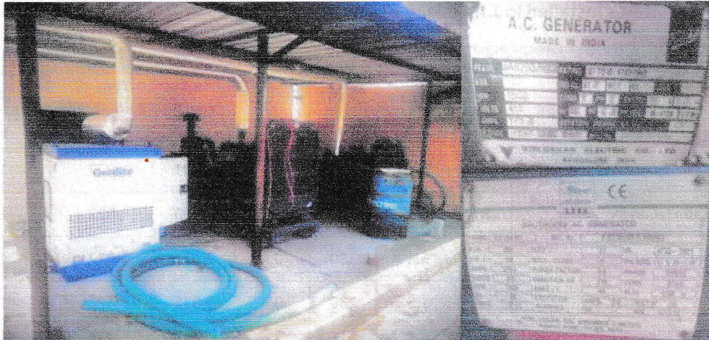
Figure 2.2.3: Diesel Generator Sets & Name plates at J.J. College of Arts and Science
